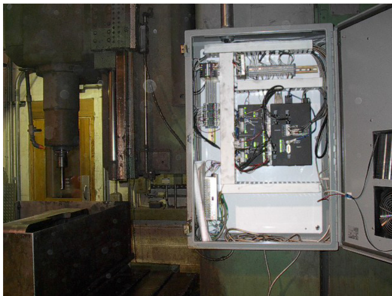
New CNC Enclosure
